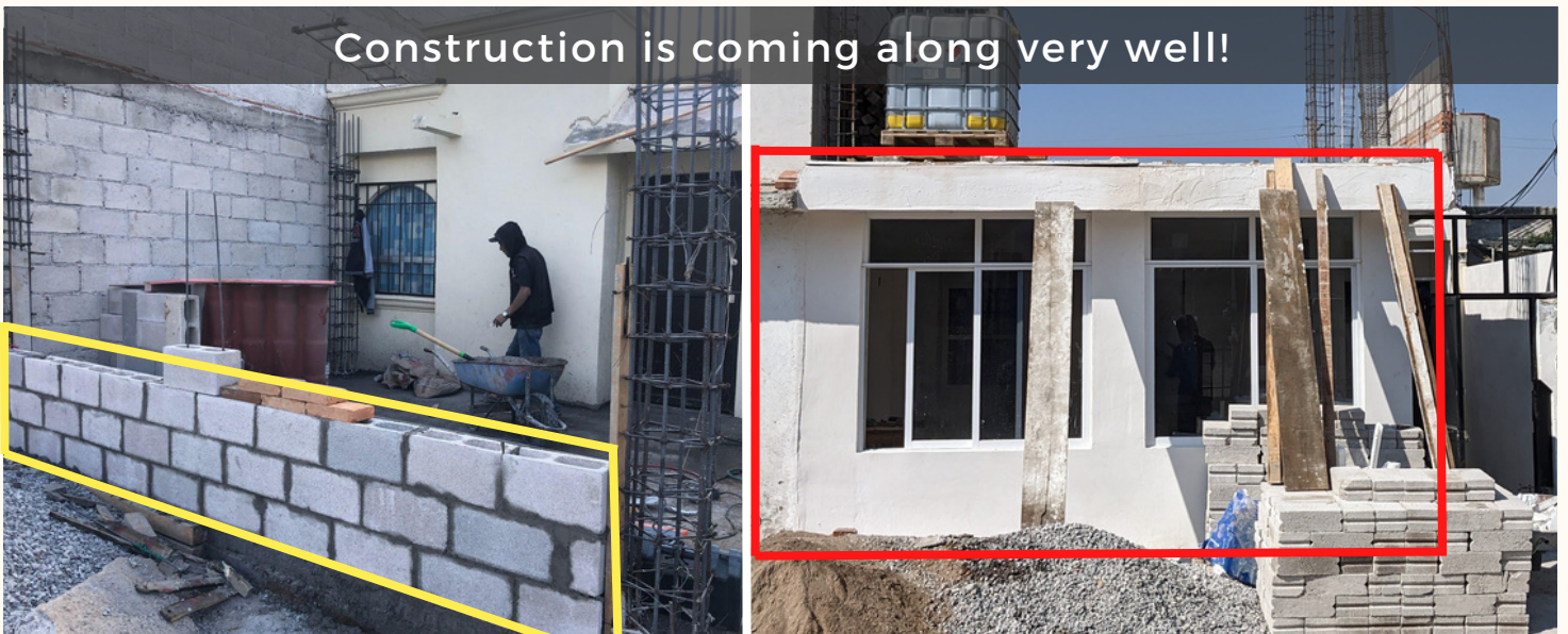
Pic #1: Yellow box shows wall being built Pic #2: Red box shows same wall with windows & room roofed in!
